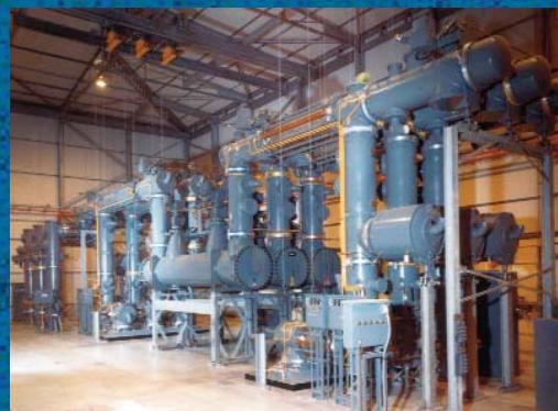
Compressed air dryers
